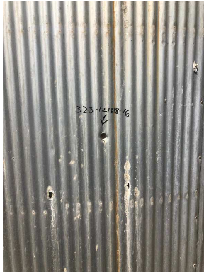
General View Sampling Point #16, TSI Tower #5, East Side.
