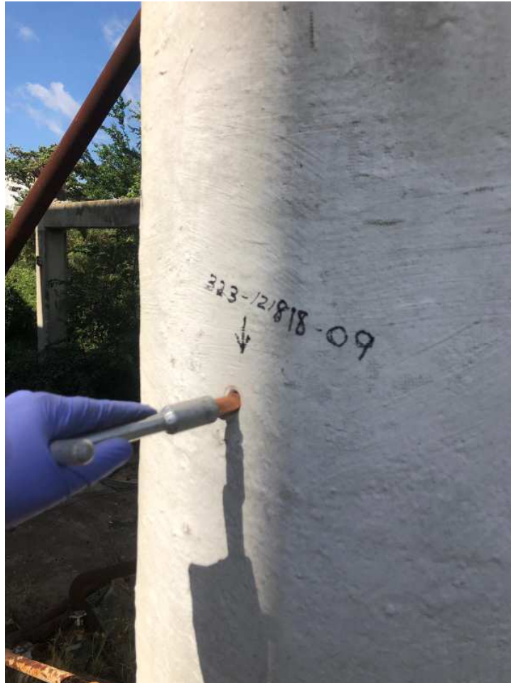
General View Sampling Point #9, TSI Tower #3, Distillation Unit North Side.
