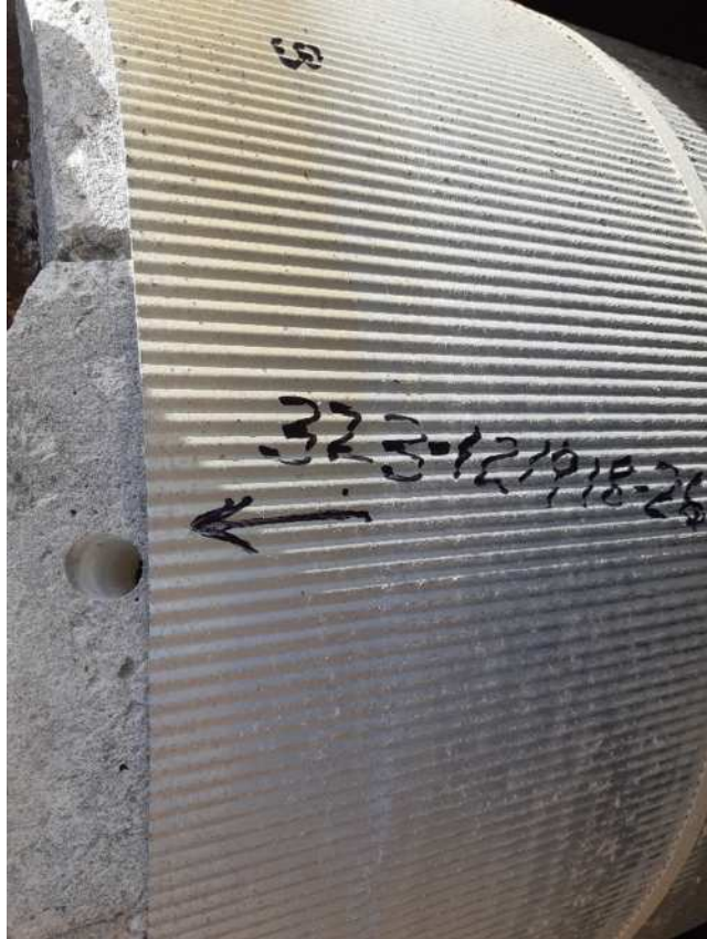
General View Sampling Point #26, TSI Interior Pipe 24'' \phi , Southeast Side.
