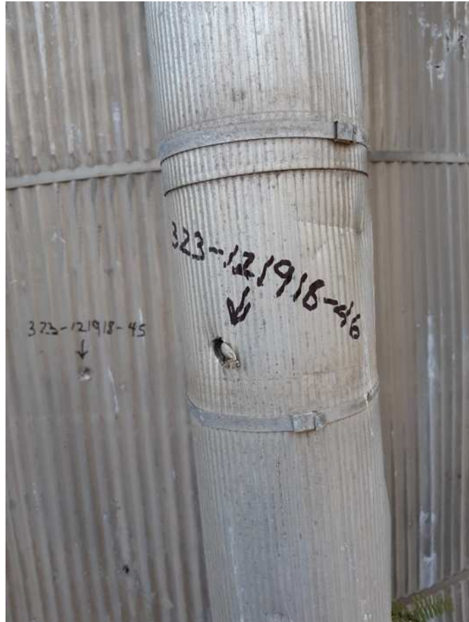
General View Sampling Point #46, 8'' \varnothing Pipe, Tower 10 TSI, Northeast Side.
