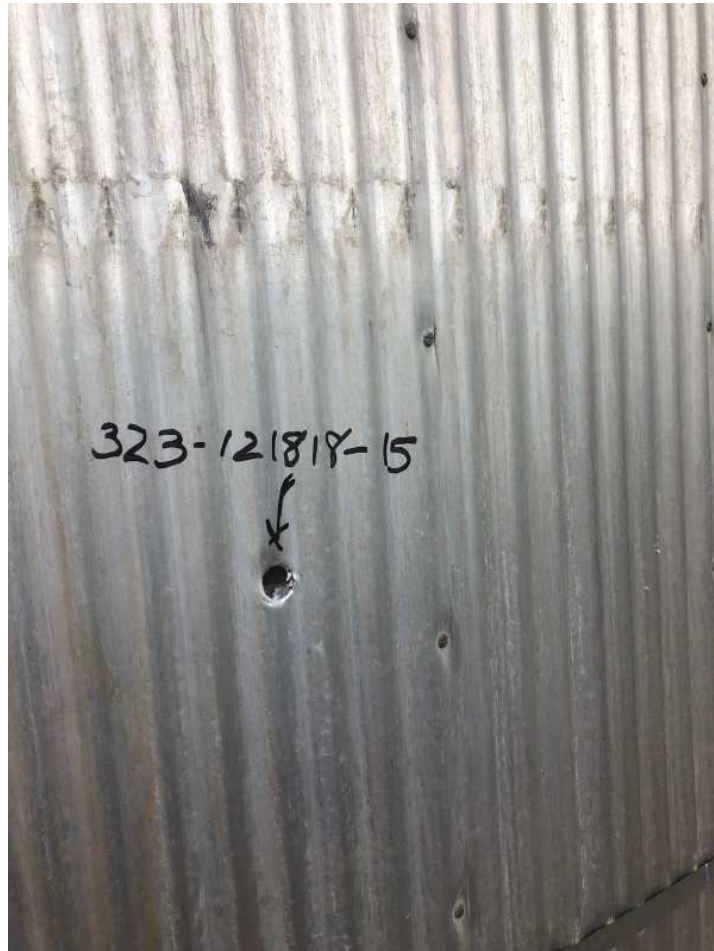
General View Sampling Point #15, TSI Tower #5, North Side.
