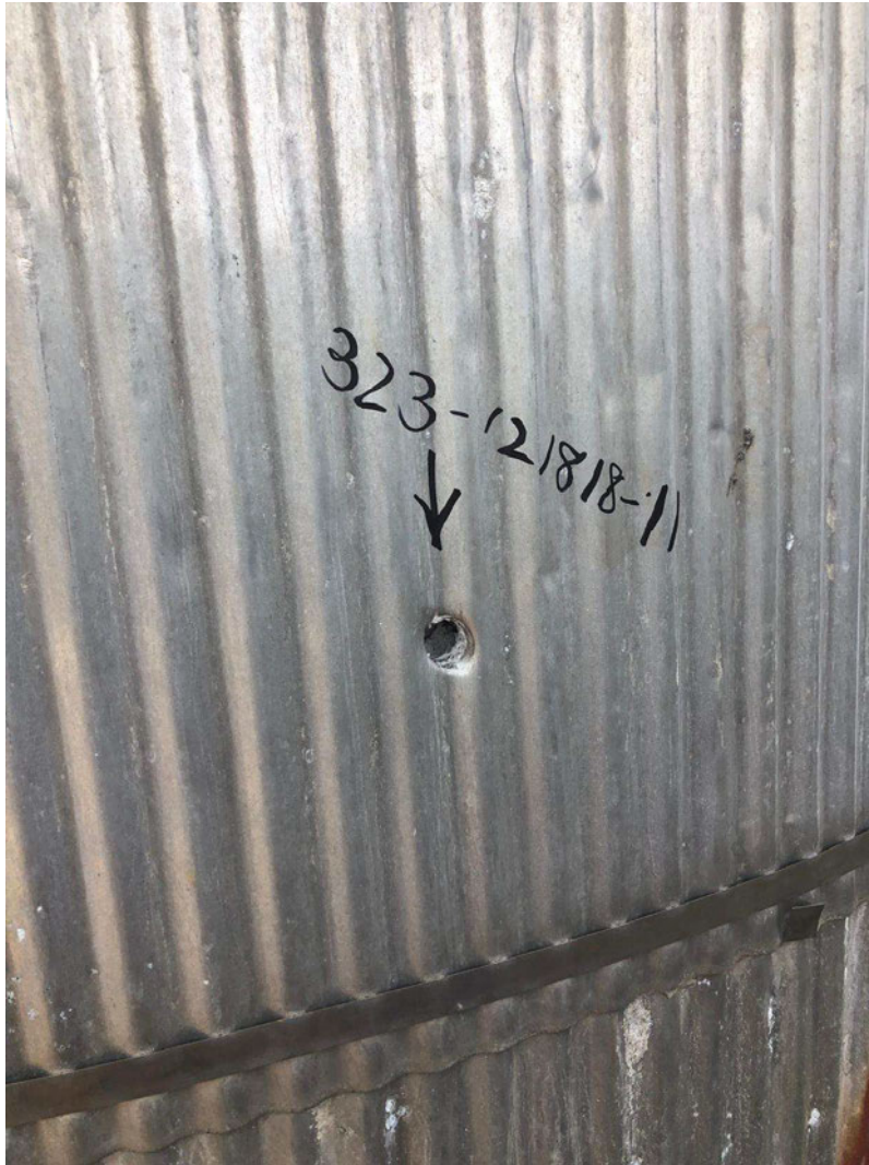
General View Sampling Point #11, TSI Tower #4, North Side
