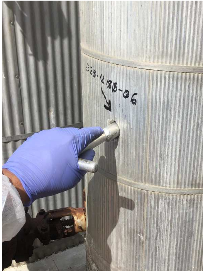
General View Sampling Point #6, TSI Tower #2, 12'' \varnothing Pipe, Northeast Side
