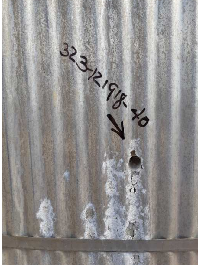
General View Sampling Point #40, Tank 6 TSI, West Side.
