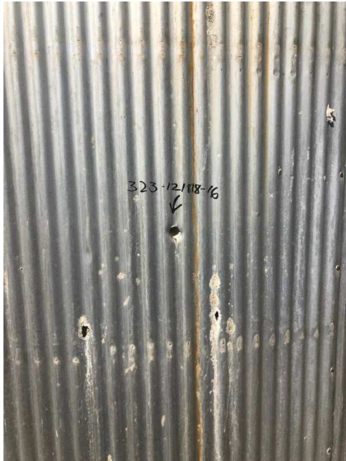
General View Sampling Point #15, TSI Tower #5, East Side.
