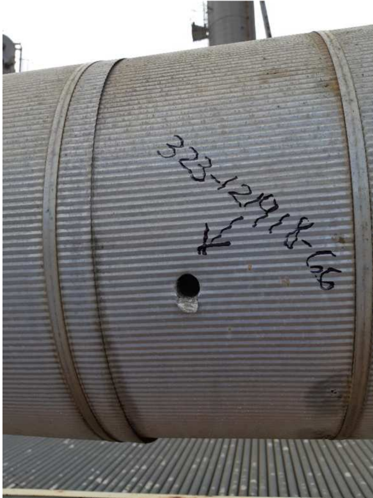
General View Sampling Point #66, Pipe Insulation 12'' \phi , Fin Fan Air Cooler
