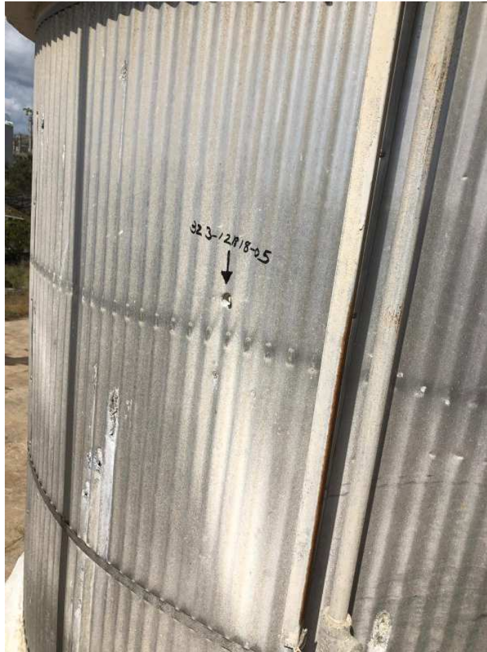
General View Sampling Point #5, TSI Tower #2 East Side
