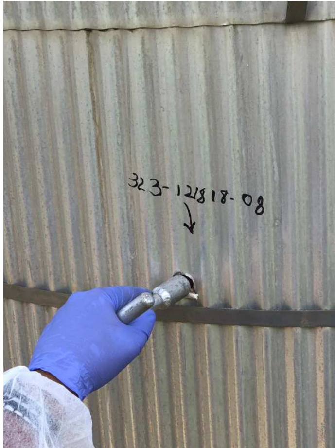
General View Sampling Point #8, TSI Tower #3, North Side.
