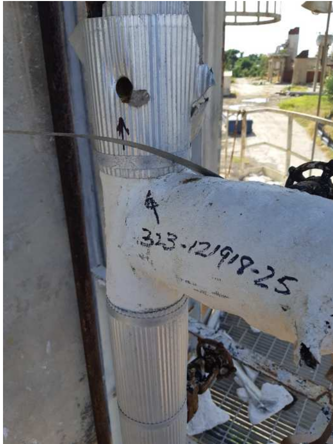
General View Sampling Point #25, TSI Tower 7, North Side.
