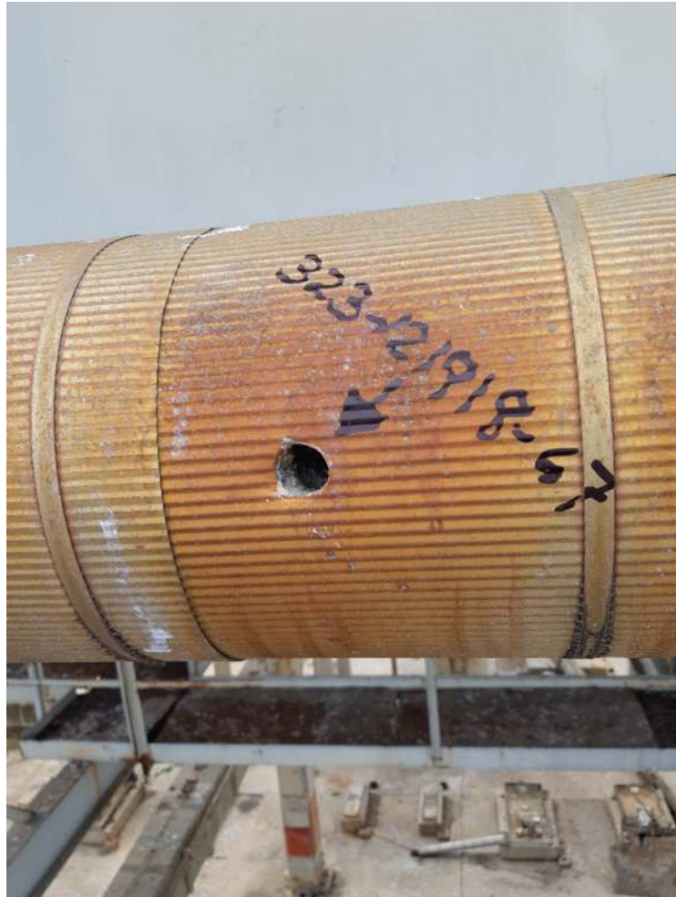
General View Sampling Point #67, Pipe Insulation 10'' \phi , Fin Fan Air Cooler
