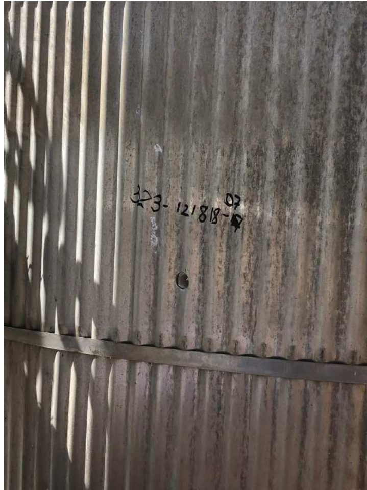
General View Sampling Point #7, TSI Tower #2, North Side.
